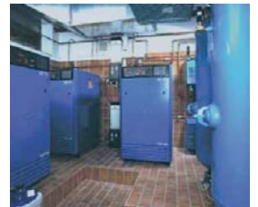
Compressed air systems: drier monitoring to avoid damage caused by humidity
