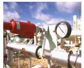
Gas engineering: humidity causes damage and reduces the value of the gas in the system
